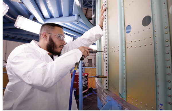
Easily fabricated drill fixtures speed the assembly process on this space launch vehicle.
